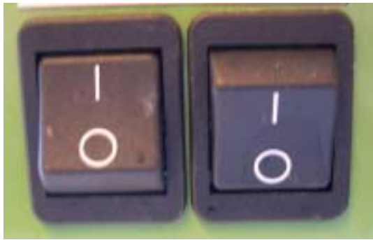
Figure 14: Pump is off now
